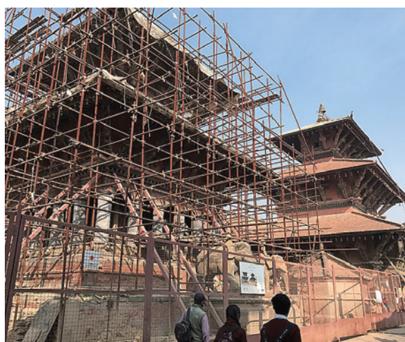
Figure 2. Damaged temples in Patan Durbar Square (November 14th, 2017 photographed by the author)
